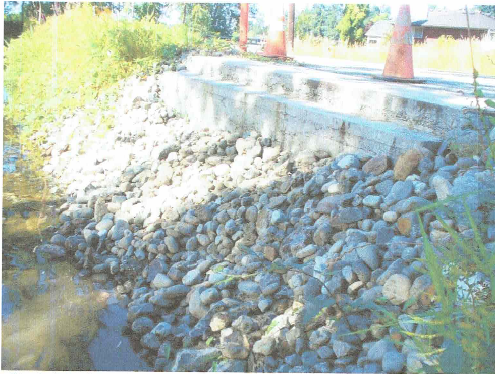
Photo #1 – Left Bank Bridge Footing and Cobbles (photo taken by Greg Johnston on 7/20/21)
